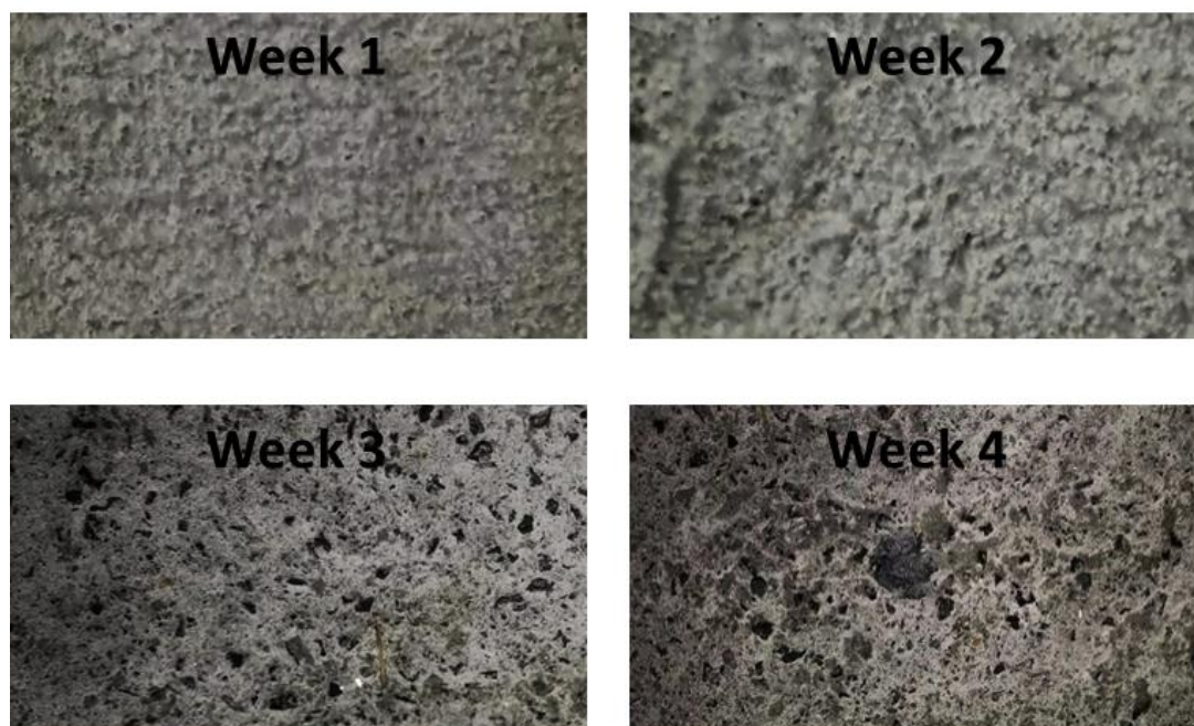
Figure 2. Repair of the surface of the concrete test specimens at different times.
