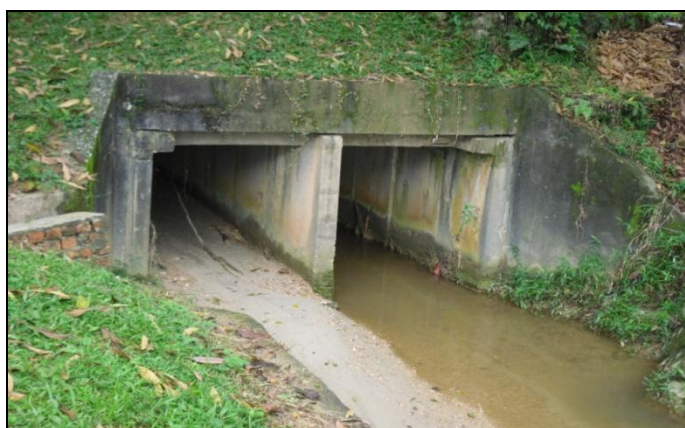
Figure 9. Monsoon drain polluted by sedimentation from construction.
